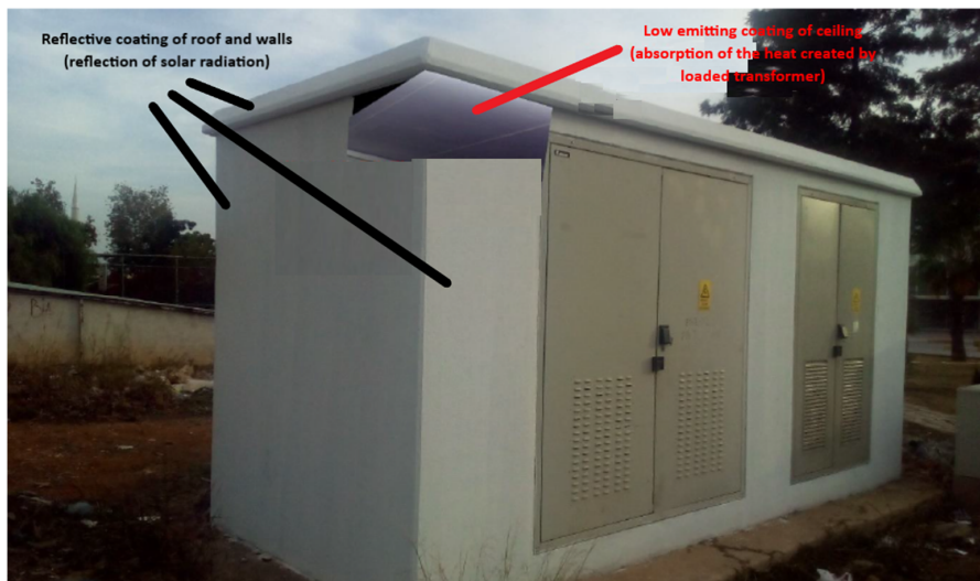
Figure 1. Sample transformer building with the reflective and low-emitting coating.
