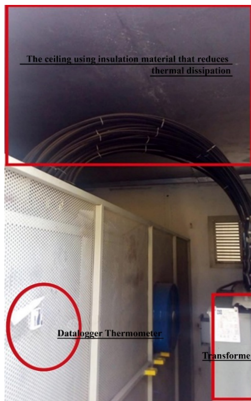
Figure 2. Location of the data loggers in the transformer building.
